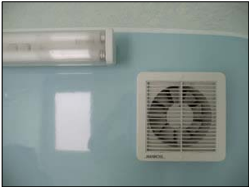
Fan and Fluorescent Lights
