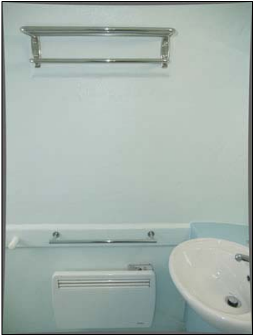
Panel Heater / Towel Rails / Vanity
